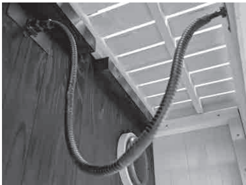
Heater Power Cable
