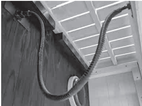
Heater Power Cable
