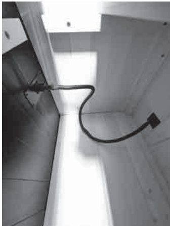
Heater Power Cable
